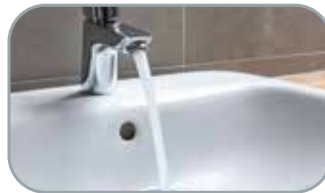
Sinks and taps
